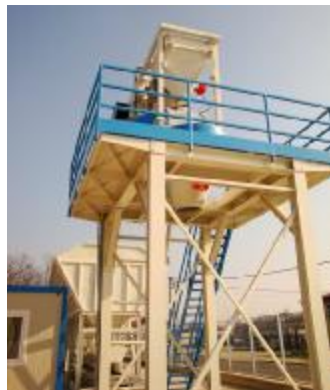
Mixers on support platform
